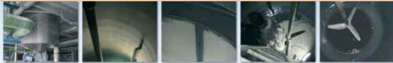
Mechanical removal of rusted patches and drying of inner surface Abrasive blast to surface profile of 75 µm and surface cleanliness SA 3 Application of Loctite® 7227 on weld lines Full surface coated, then after partial cure the second coat was applied After 24 hrs, the tank was ready to be filled
