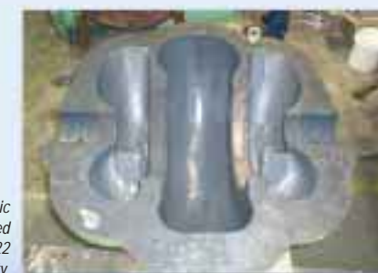
Loctite® Nordbak® 7227 Brushable Ceramic Grey applied to seal the blast. Fill the corroded and abraded areas using Loctite® Wear 7222 Resistant Putty.
