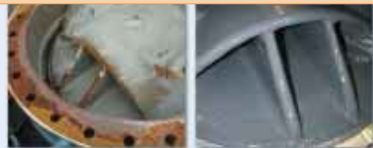
The corroded butterfly valve – before and after repair
