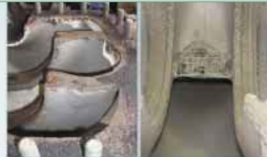
Pitting and erosion was clearly evident
